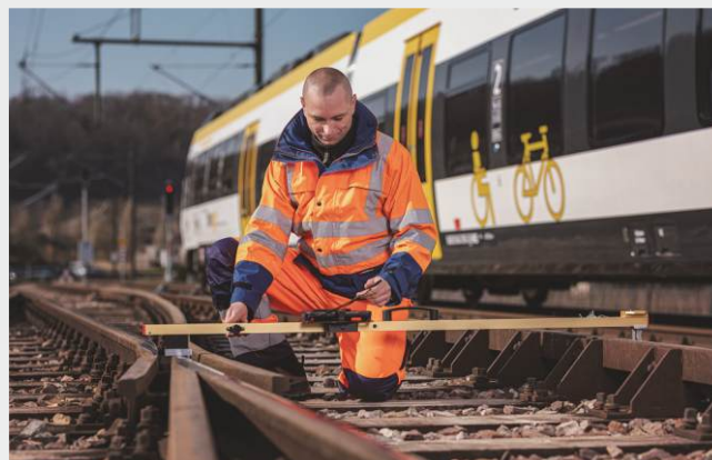
Track and switch inspection system MessReg PTP II
